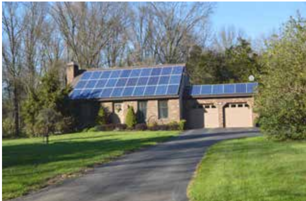
An example of a residential home with rooftop solar panels in Upper Frederick Township.
