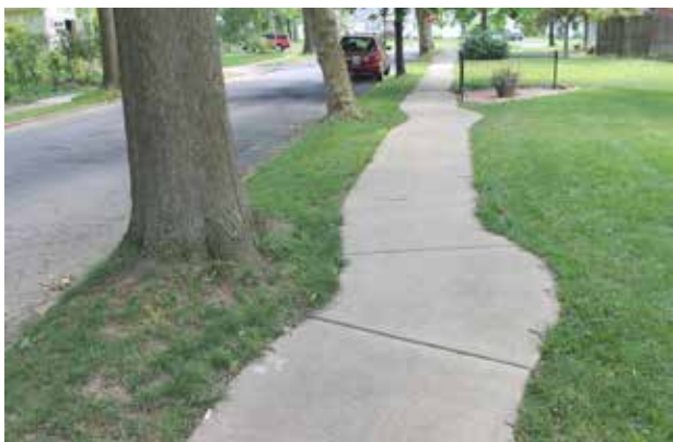
Sidewalks can be repaired and moved away from tree roots to minimize future damage.
