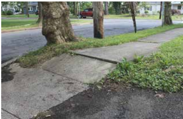
Mature tree roots create uplift in the sidewalk and impair pedestrian safety.
