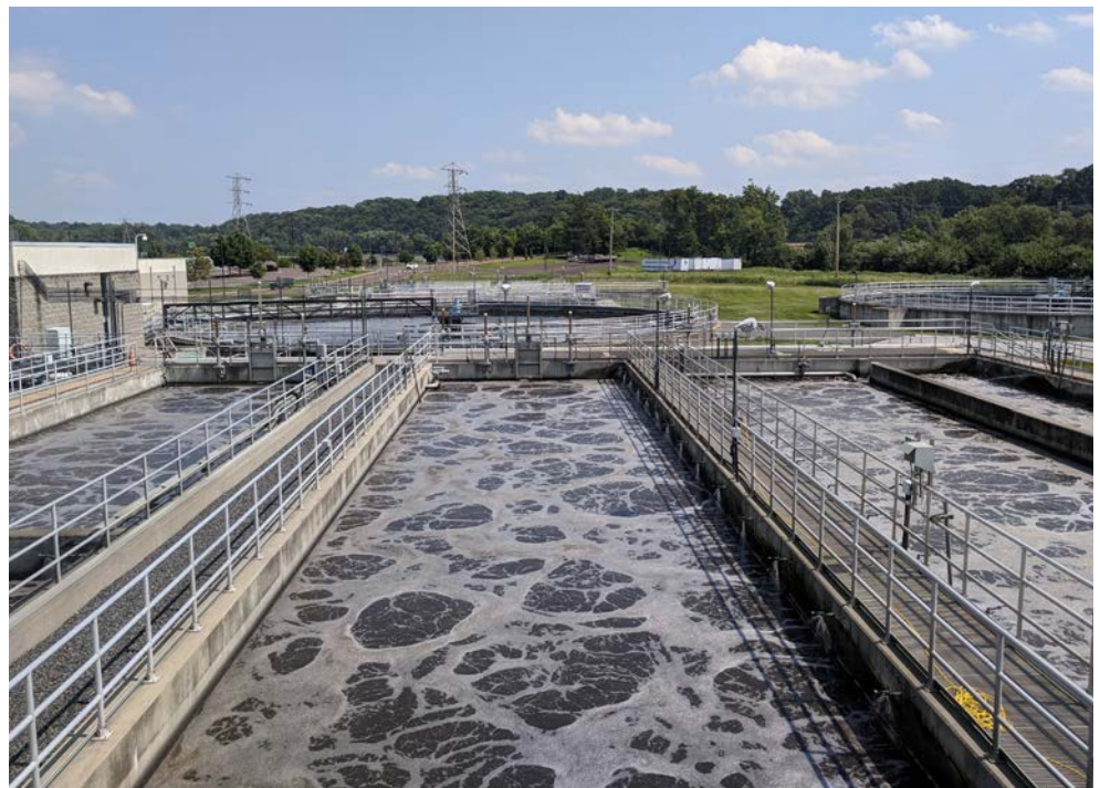
Aeration Tank, Oaks Wastewater Treatment Plant, Upper Providence Township
