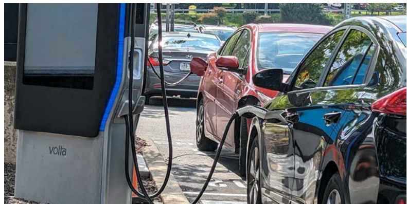
EV charging station installed in a grocery store parking lot, Upper Merion Township
