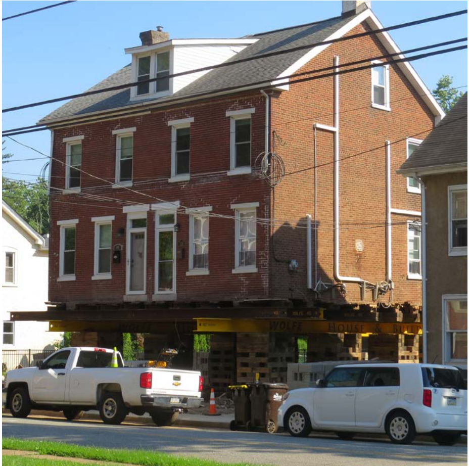
A residence being elevated as a resiliency measure after incurring flood damage during Hurricane Ida, Upper Providence Township
